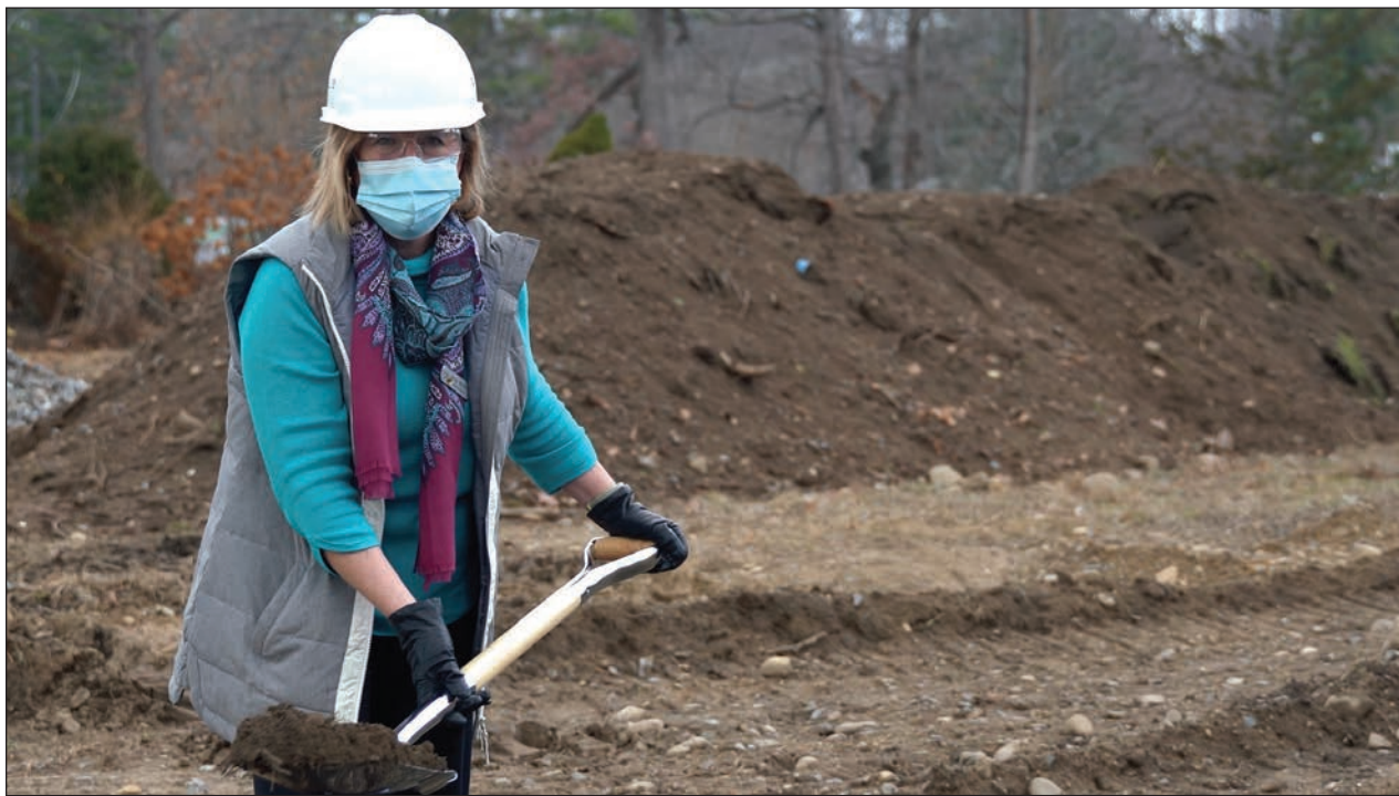
Peabody Home Executive Director Meg Miller at the groundbreaking for the comprehensive new senior living facility.
