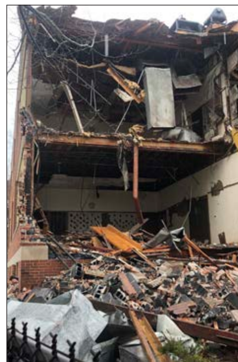
More of the former classroom space can be seen during the demolition.
