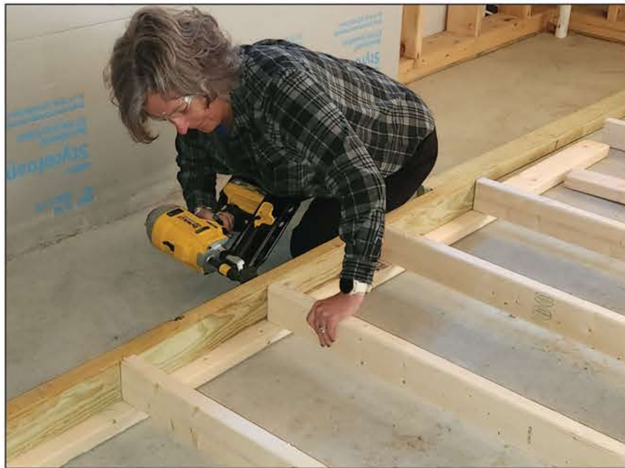
Board member Patty O'Neill wasn't so sure of the nail gun during her visit to Pemi Valley Habitat's new home build in Sanbornton recently, but was a quick learner.
