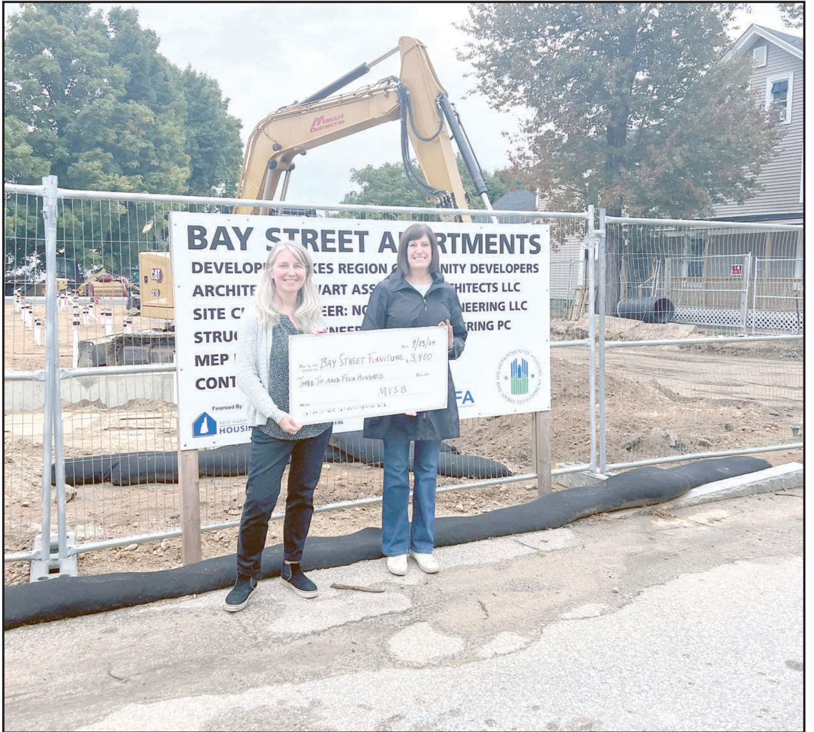
From left, Carmen Lorentz, Lakes Region Community Developers Executive Director, and Lori Borrin, MVS VP Mortgage Loan Officer NMLS# 165814 and LRCD Board of Directors Treasurer, stand at the site of the Bay Street Apartments in Laconia, which is currently under construction and set to open in spring 2025.
